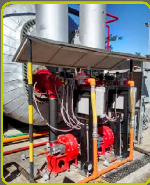
Reactores de Gas
